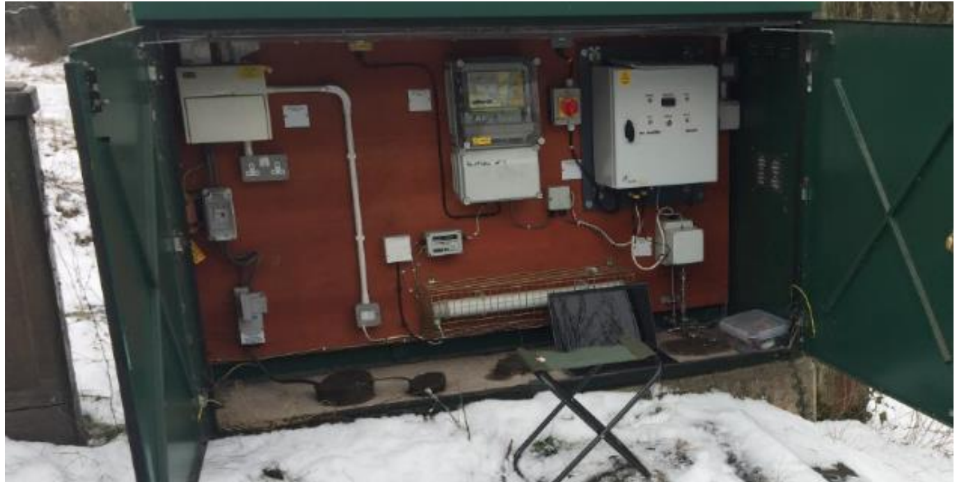
Unit installed in a cabinet. There are 6 of these cabinets on the industrial estate and include heating system, lighting protection and connection to the telemetry system.
