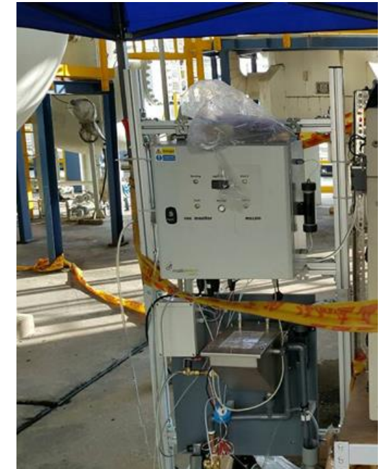
Photo showing the MS1200 in the petrochemical plant.
