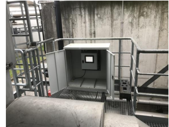
A picture of the unit installed in the cabinet for further weather protection
